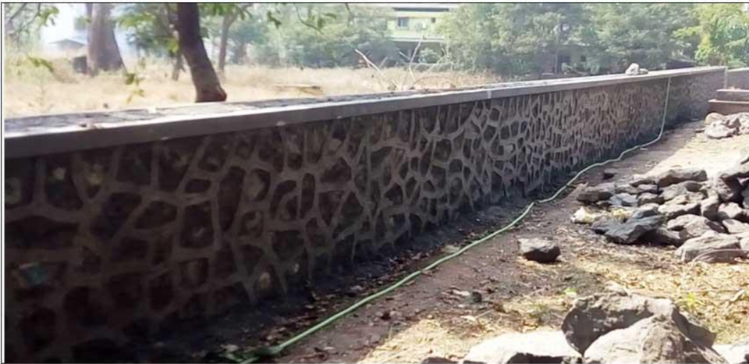
Paid for bothside Compound wall civil construction work with Material of Rs.18,71,201/- at Arjun Kanu Bhoi Hutatma Smarak Nangalwadi.
